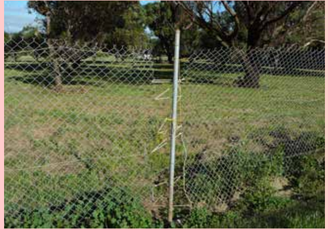
Damaged, inadequate fencing
