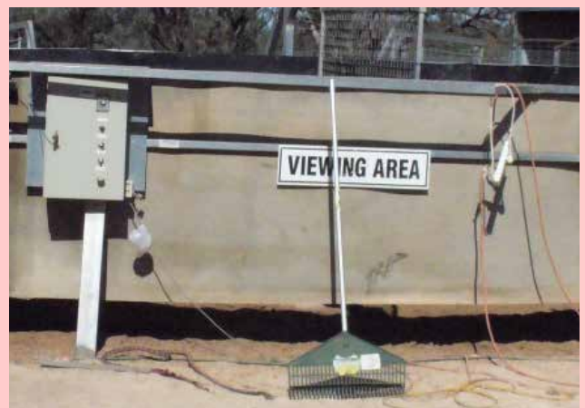
Unsafe scenario with a temporary power board being used and leads hanging down
