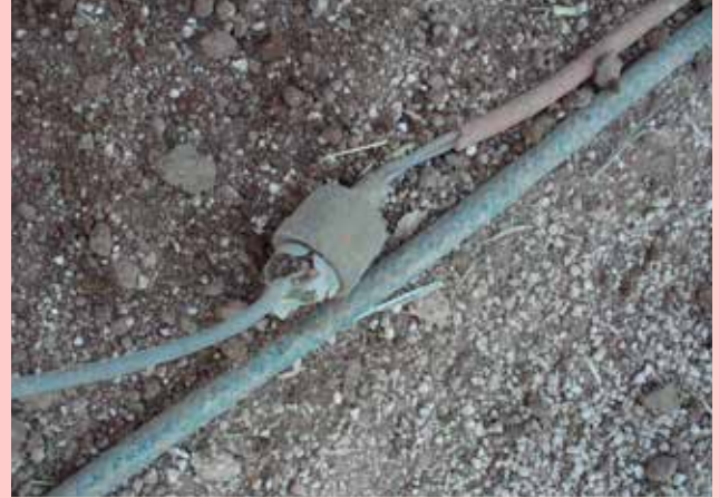
Damaged power leads, which haven't been inspected and tagged, shouldn't be used
