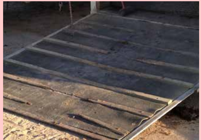
Hazardous surface that may cause trips and falls
