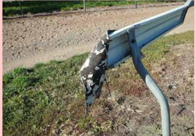
Rails not maintained
