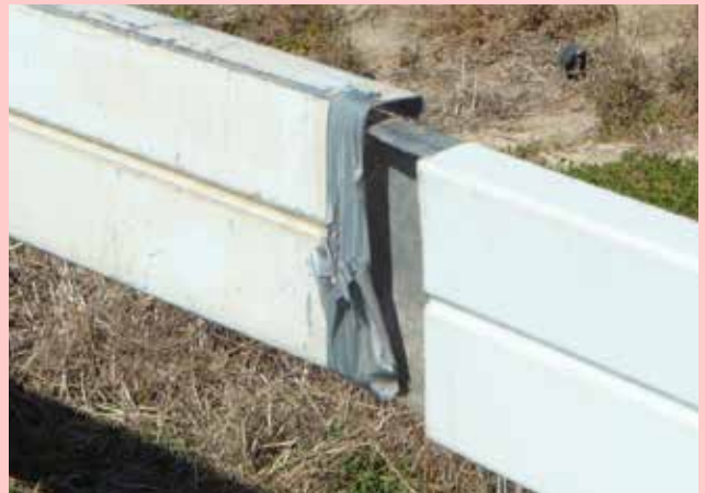
An unsatisfactory attempt to maintain rails using tape
