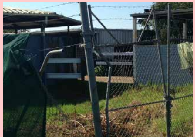
Damaged fence providing inadequate security
