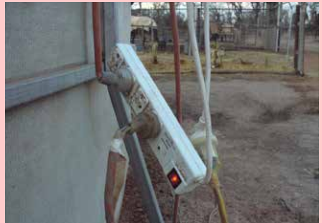
Portable power leads shouldn't be used permanently instead of fixed wiring
