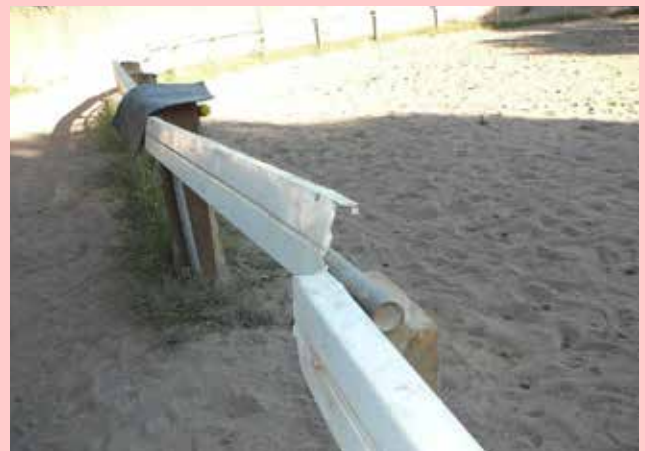
Unsafe scenario where rails are damaged, with sharp edges protruding
