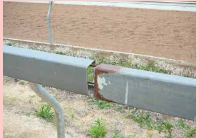
Damaged railing is a health and safety risk to horses and riders
