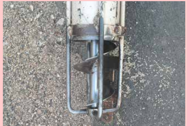
Auger screw shouldn't allow people to easily access the rotating component by putting their hands through the guard
